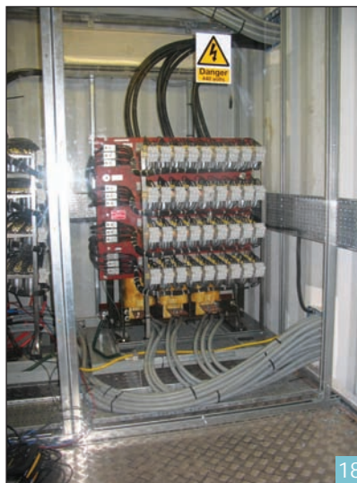
One of two 750-kW wide-spectrum harmonic filters installed on each group of combined thruster and pump load.
