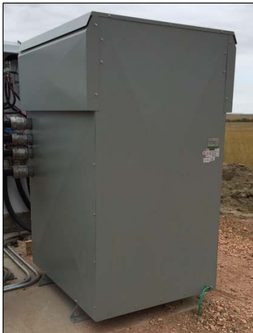
Fig. 16 1100 HP Sinewave Filter Installation
