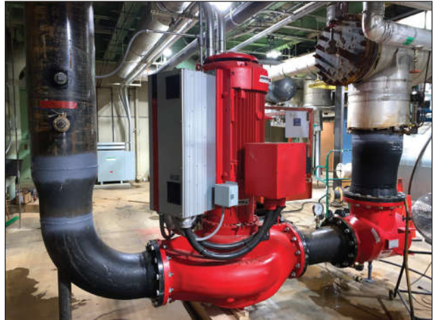
400HP Chilled Water Pump with Pump Mounted Variable Frequency Drive
