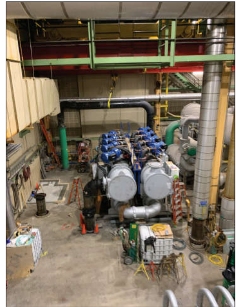
3200 Ton Chiller installed at RED Rochester's Building 87
