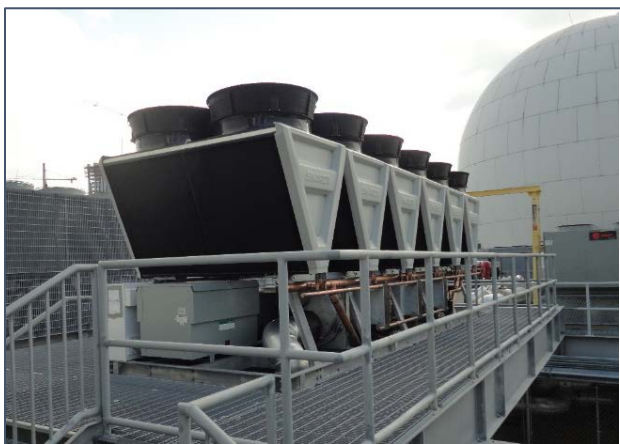
Fig. 1: Rooftop Air Handler
